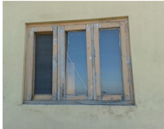
Damaged window of Tuck Shop
