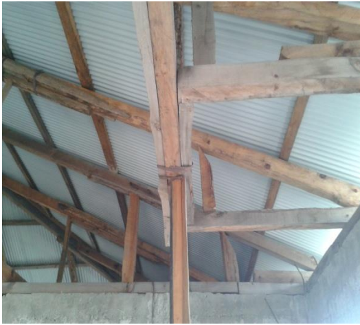
Broken horizontal member supported by wooden log
