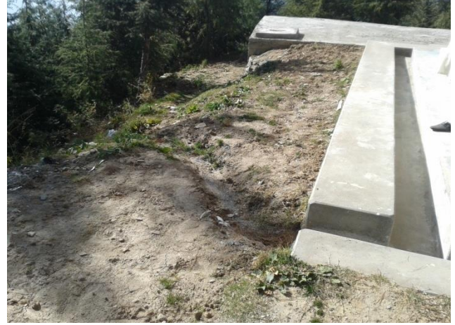
Area in front of Rest House Needs Soil Stabilization
